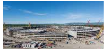
Existing buildings on the site were demolished and the rubble recycled to make concrete for the foundations of Apple Campus 2.
