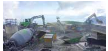
The concrete that was needed was produced locally: on the mountain itself.
